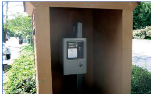
Figure 3-16: Centralized Ticket Machine, Water Street Lot
