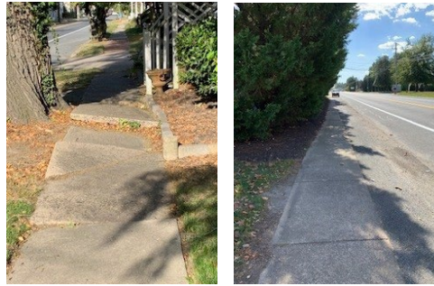
ADA Conformity Issues
